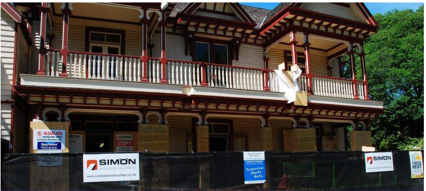
Repairs to Riccarton House began in October 2012 and are scheduled for completion in early 2014.
